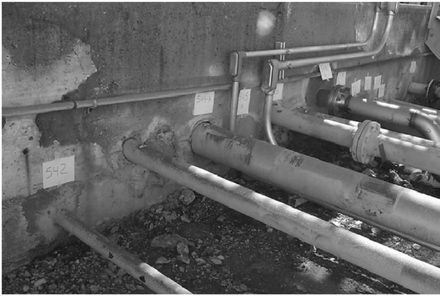
FIG. 1. Example of applications where the areas of concern are not directly accessible: regions of pipelines embedded in concrete.
